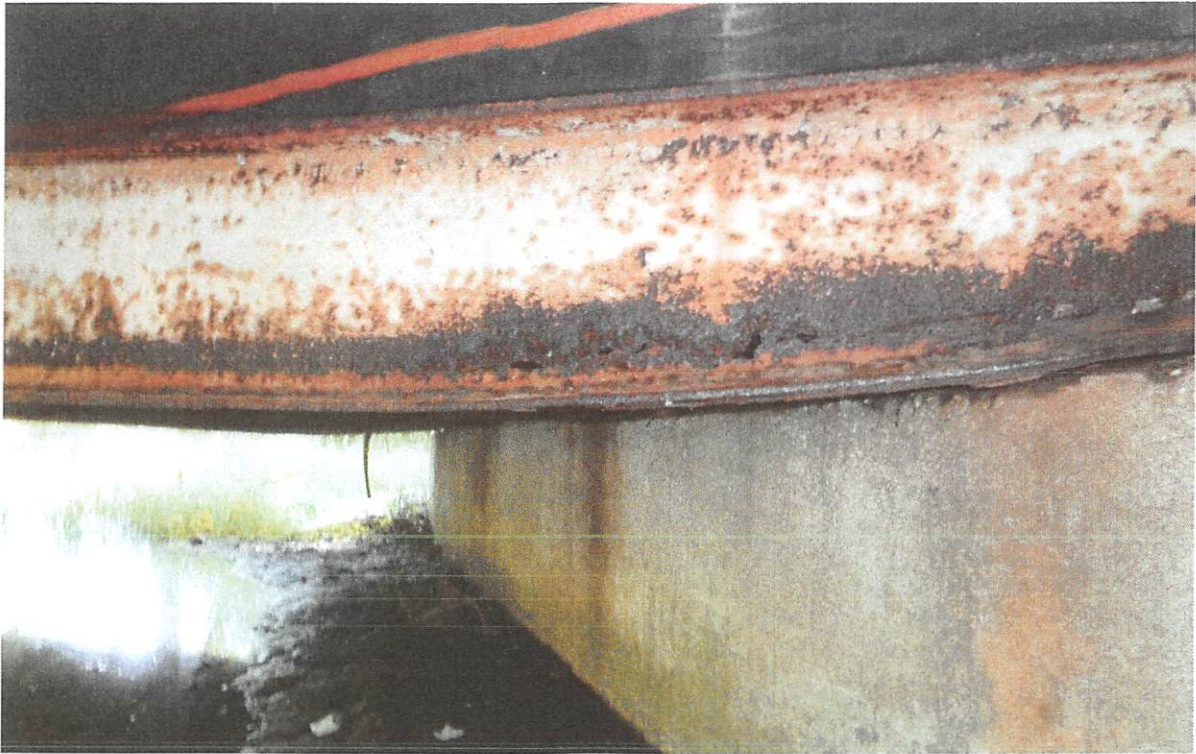
Photograph 3 - Slotted holes along web of interior girder (B4) and significant sagging. Girder located under wheel path.
