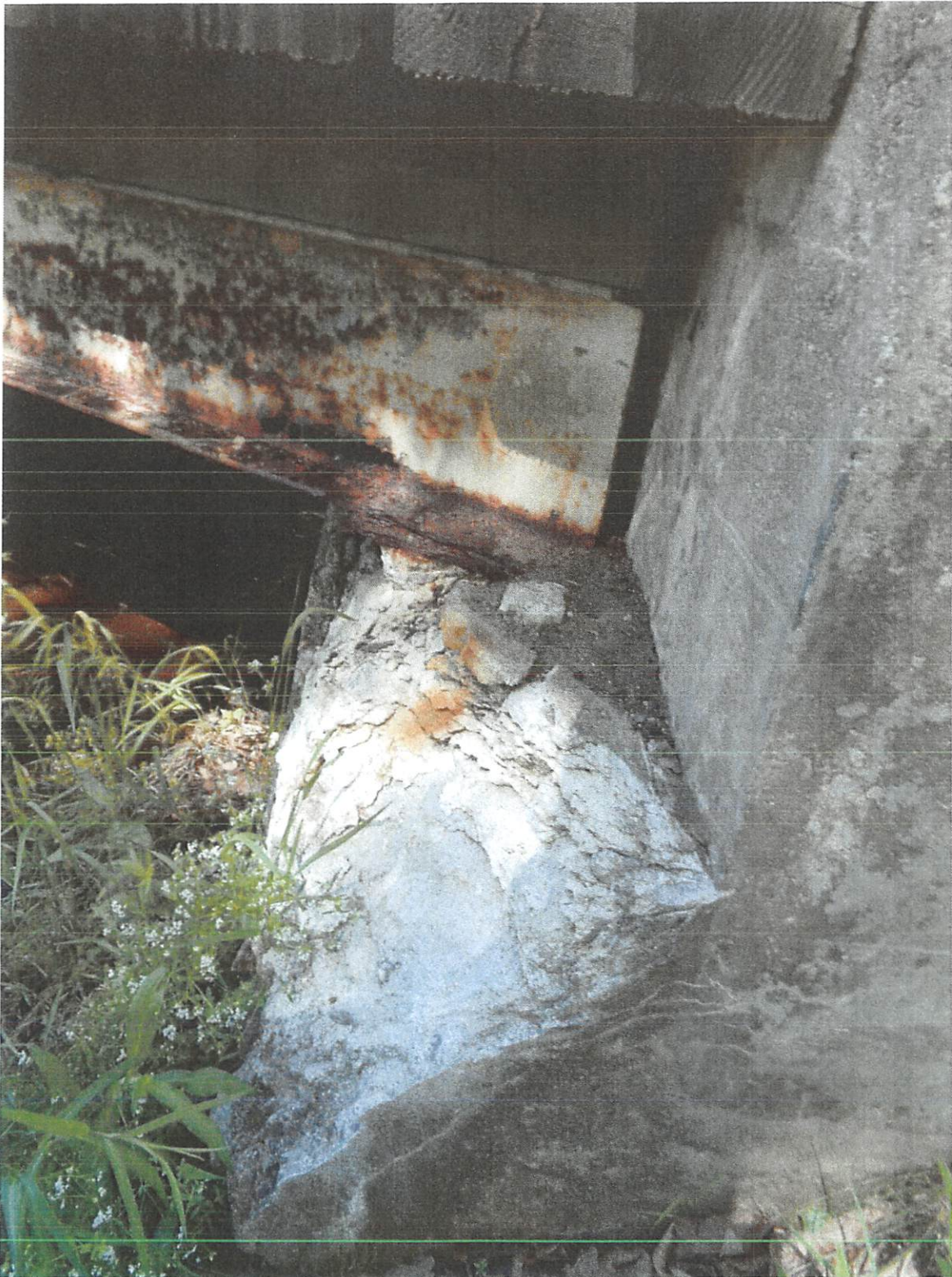
Photograph 4 - Spalling and delaminated concrete at North Abutment, hole in web of Easterly fascia girder (B1). Debris collected on abutment seat.
