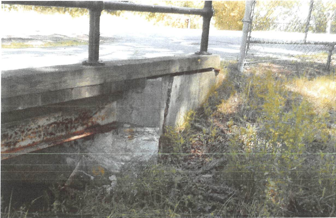
Photograph 6 - Cracked northwest wingwall, separated from abutment
